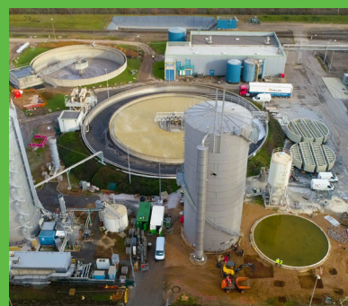
WWTP / new biogas unit
